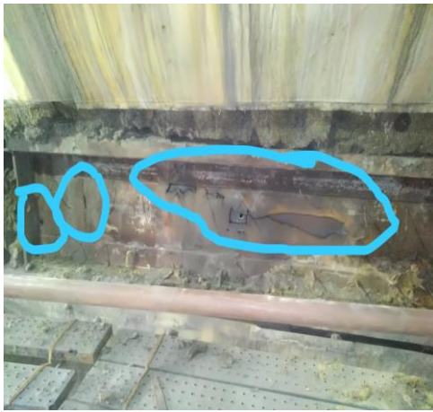
Fig10. Ingress cracks located
