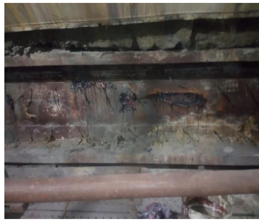
Fig 11. Air Ingress points plugged
